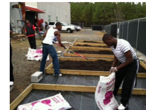
The students have installed the nursery fabric and are filling the raised beds with soil.
