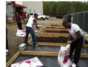
The students have installed the nursery fabric and are filling the raised beds with soil.
