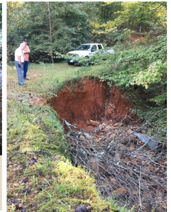
Durham County farm road crossing damaged by hurricane Florence and Michael
