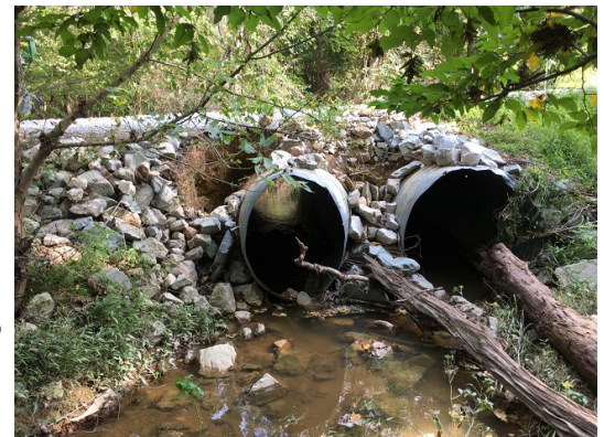
Durham County farm road crossing damaged by hurricane Florence and Michael
