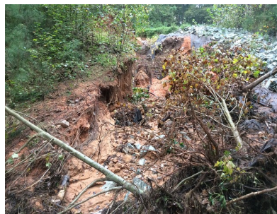
Durham County agriculture pond dam damaged by hurricane Florence and Michael
