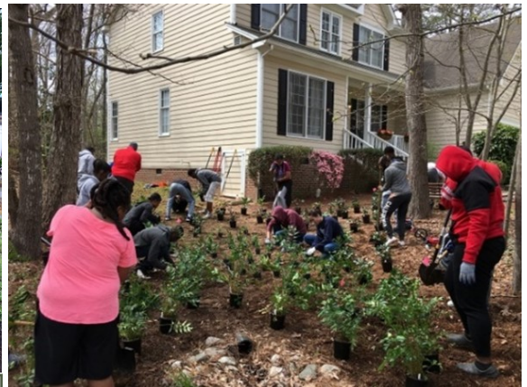
Students & teachers participating in the BETC program install a downspout disconnection and a critical area planting
