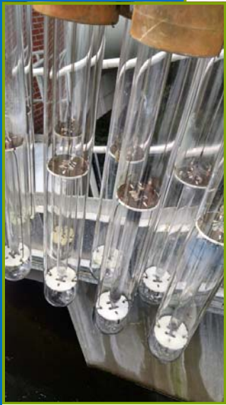
Ultraviolet (UV) Bulb System
