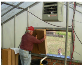
Farm Bureau Chairman, Talmage Layton helps with the installation of the Cool- Pak at Jordan HS.
