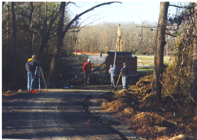
Work in 1999 on the newest section of the Rocky Creek Trail behind Shepherd Middle School
