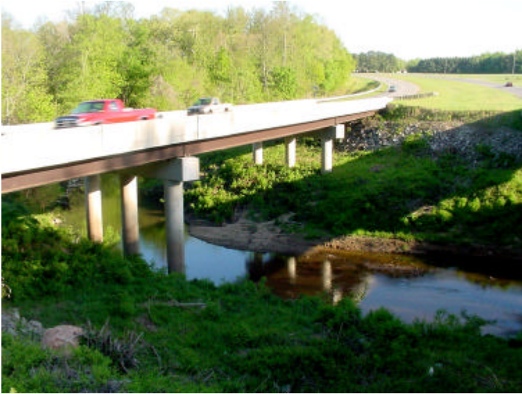
Large bridge spans over creeks and rivers provide a safe place for wildlife movement under major roadways. (Luck)
